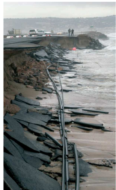
Figure 2: 139 In Thau (France), coastal erosion affecting a road located too close to the shore.
